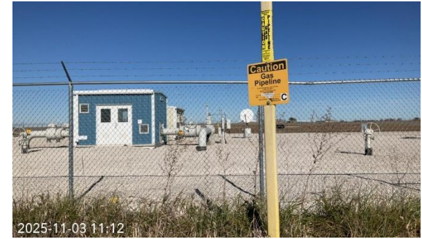
Photo 14. View of Northern's existing Ogden to Ventura pipeline valve 7 setting, photo taken facing north.
